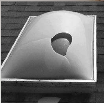
Old acrylic domes can be easily damaged
